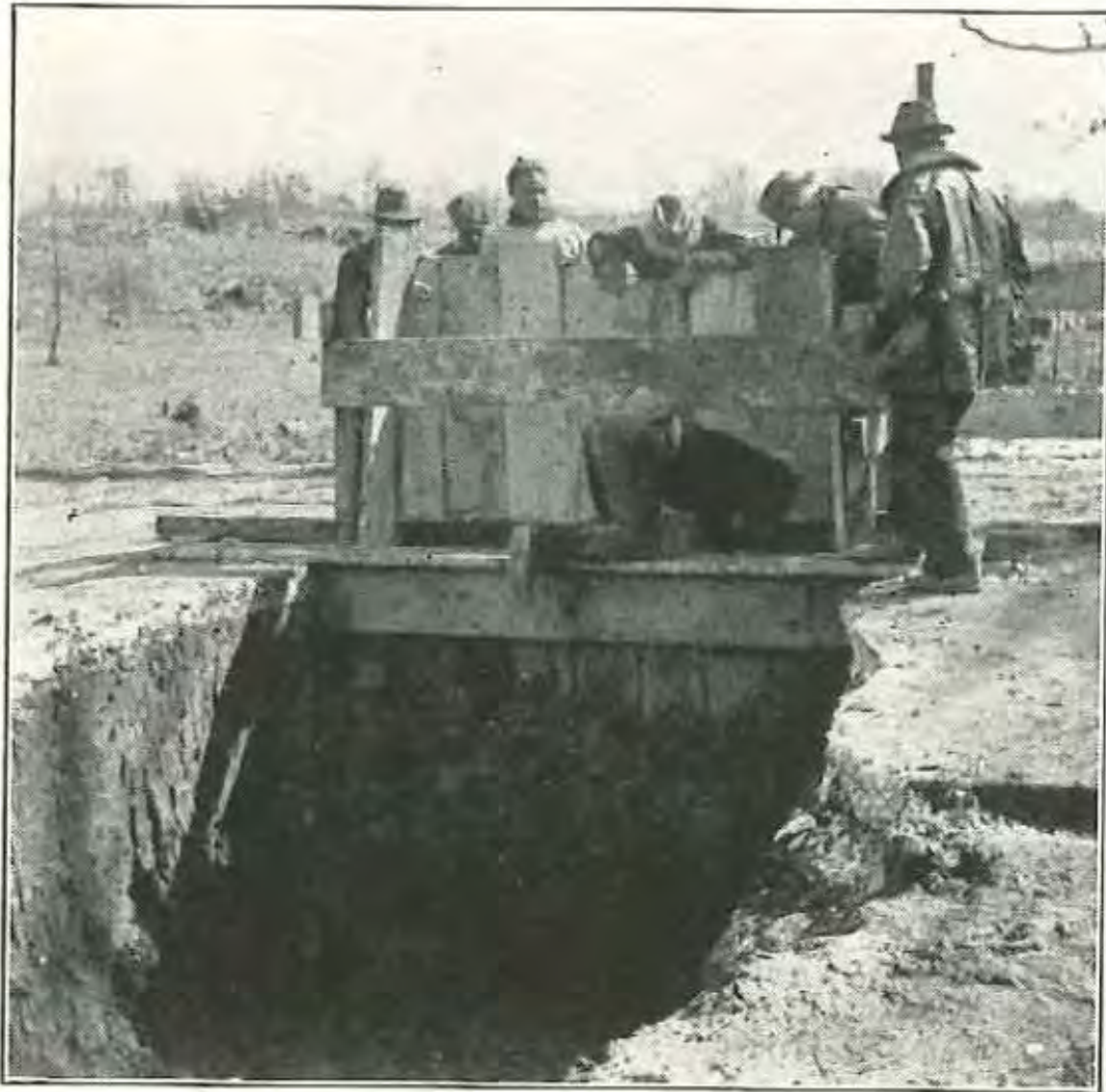
LOWERING OF CULVERT ON SPA ROAD BY STATE ROADS COMMISSION IN ORDER TO DRAIN THE UPPER REACHES OF SPA CREEK.
